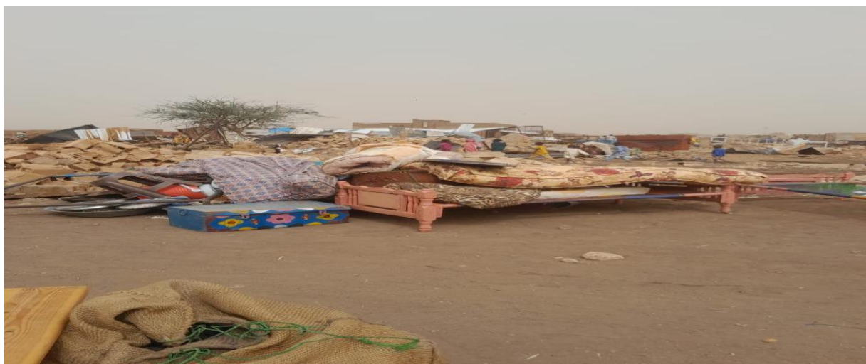
Homes demolished without allowing their residents to collect their belongings
