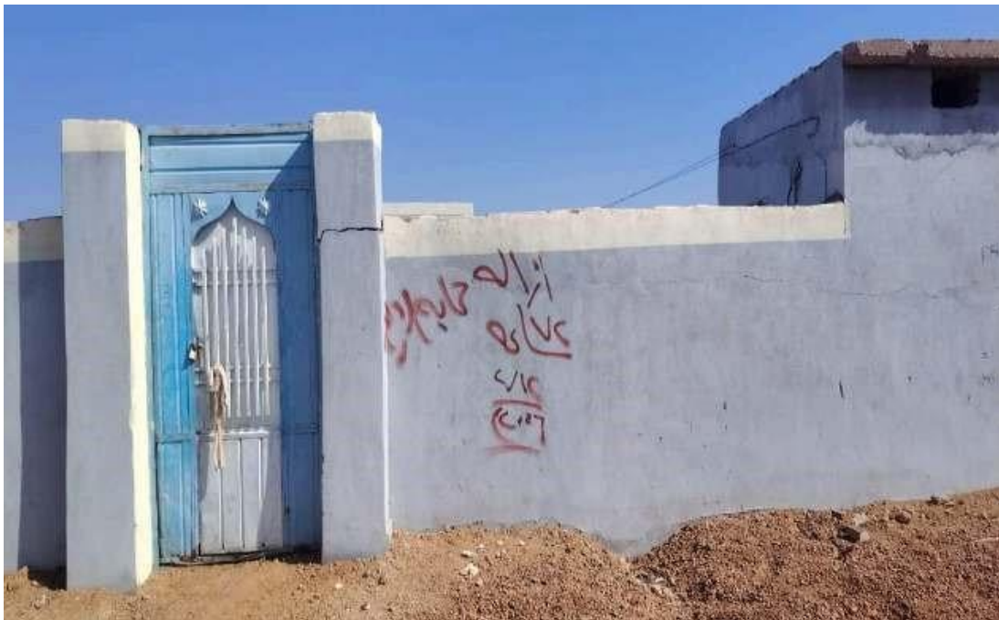
Mark on the wall of one of the inhabited homes announcing that it will be demolished by the authorities within 72 hours, Khartoum North Locality, March 2026
