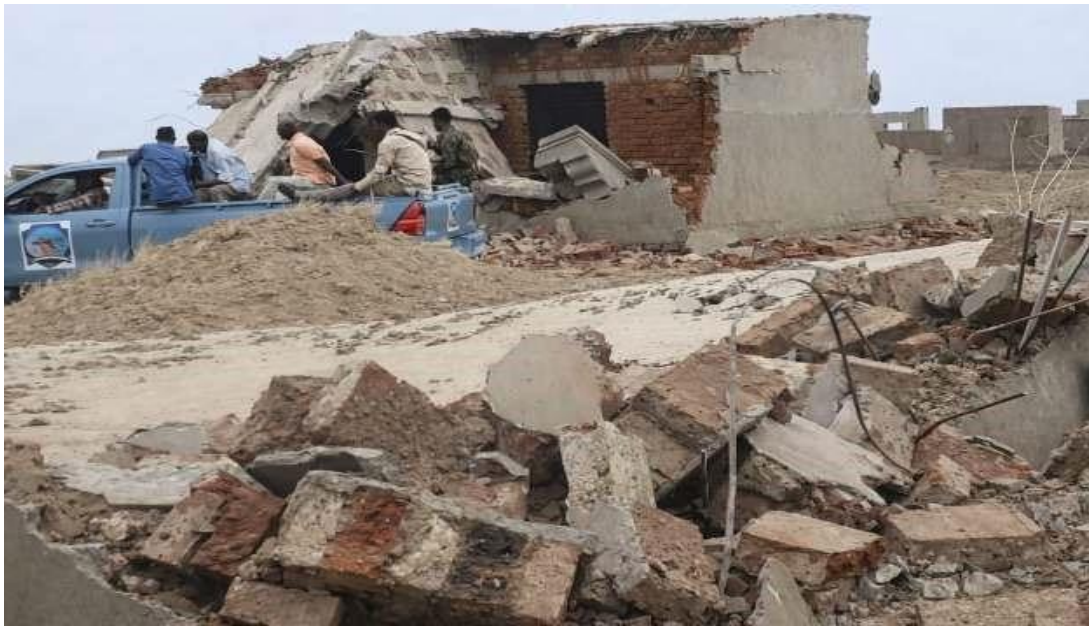
A house built with concrete construction material demolished in Khartoum North
